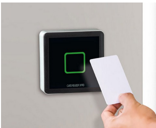
Access control system
