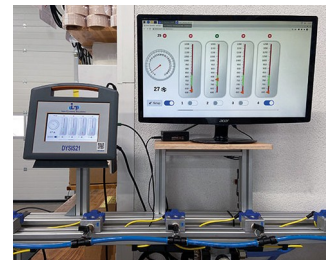
Monitoring system for cleaning nozzles
