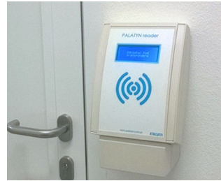
RFID access control readers
