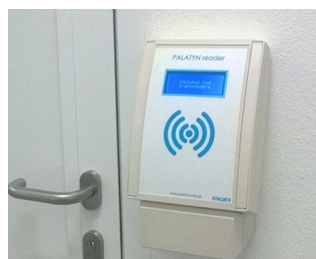
RFID access control readers
